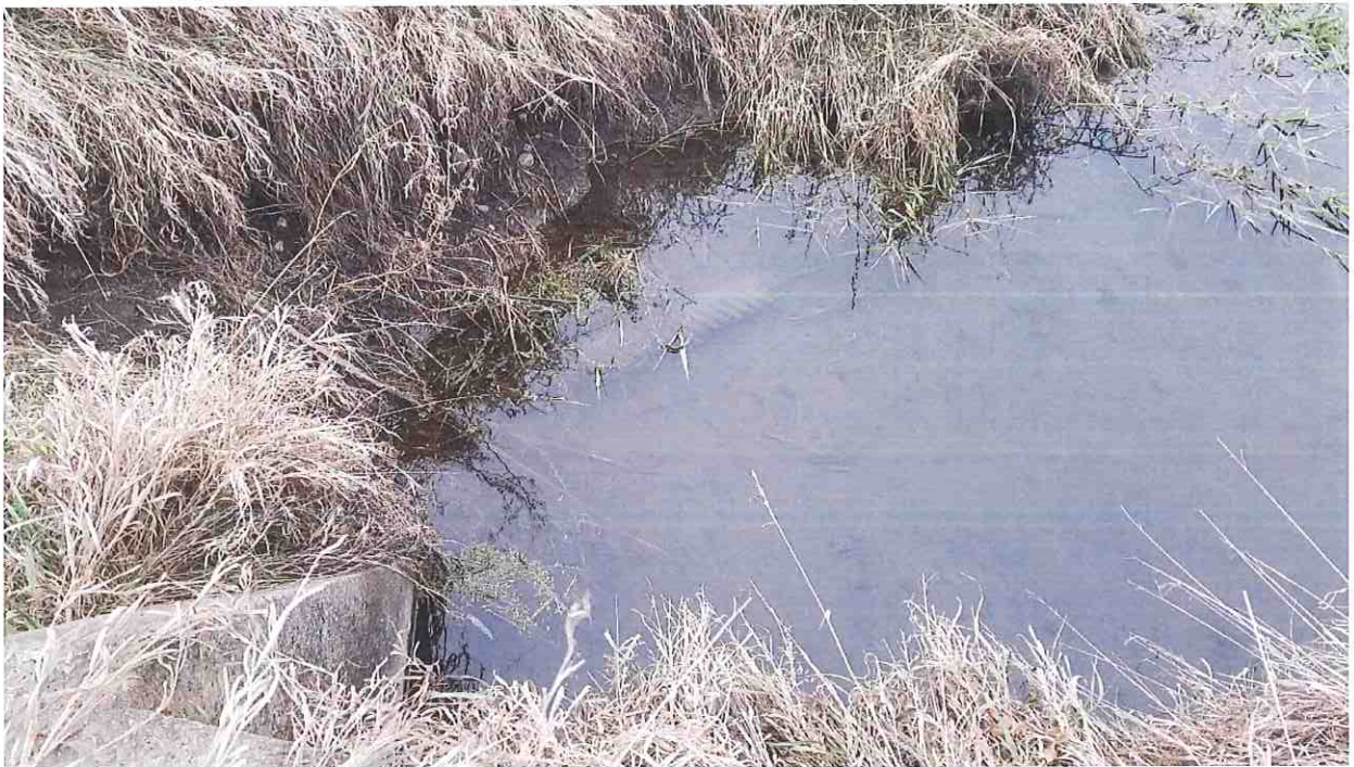
Tile outlet submerged under water at bulkhead.
