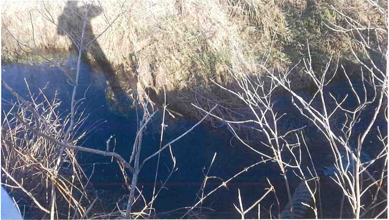
Bank sloughed into Open Ditch toward bent tile outlet.
