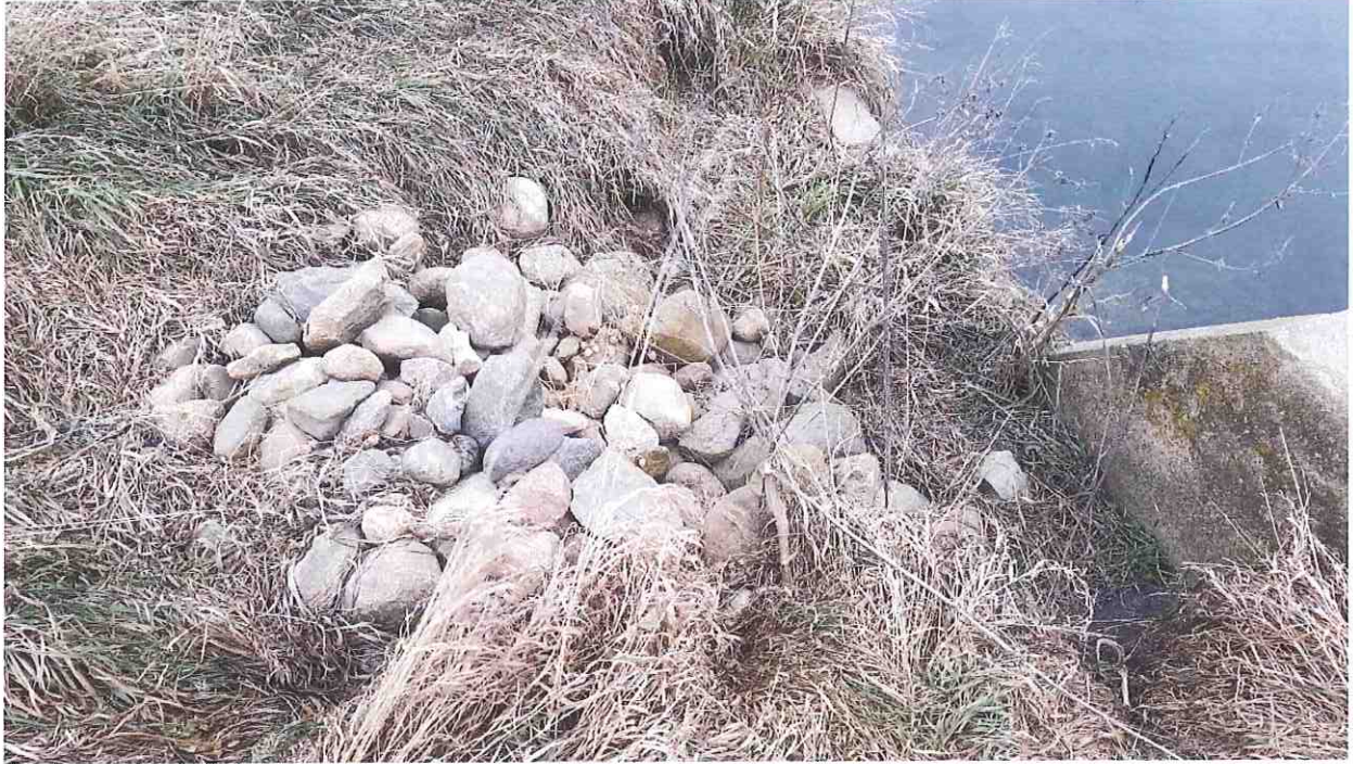
Erosion and field stone on top of bulkhead.
