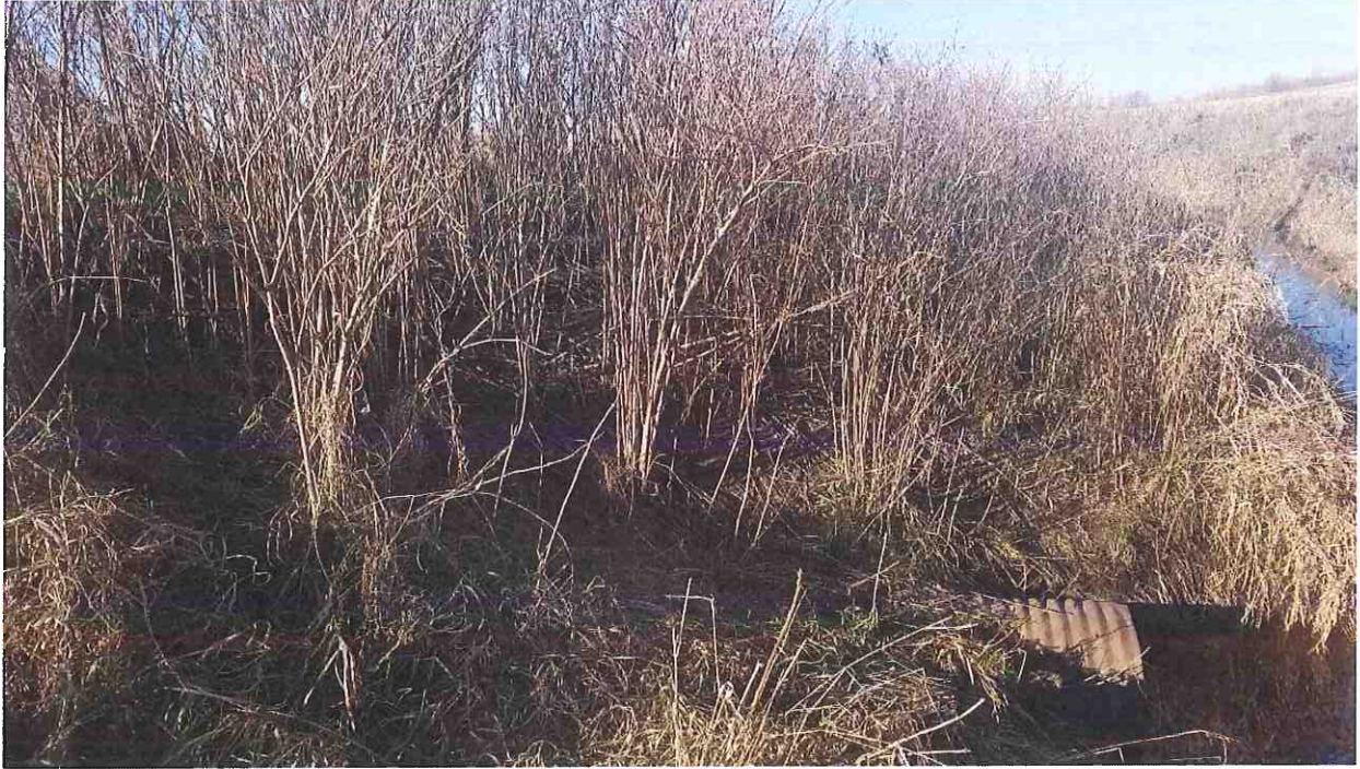
Woody vegetation and surface drain partially submerged, deformed, and rusty.
