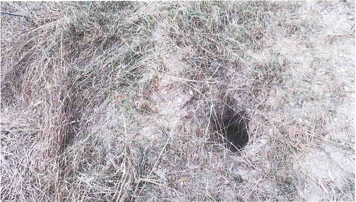
Sinkhole above Main tile on east shoulder of S Avenue.
