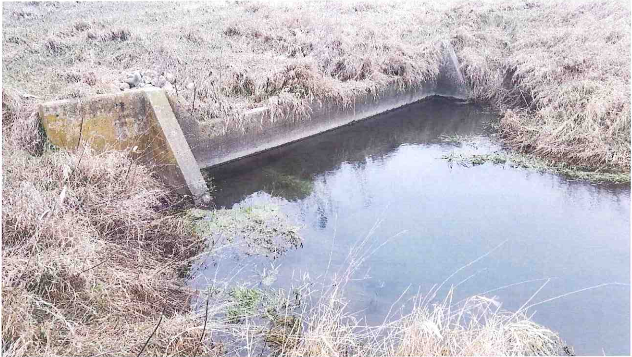
Main tile outlet fully submerged under water and not visible at bulkhead.
