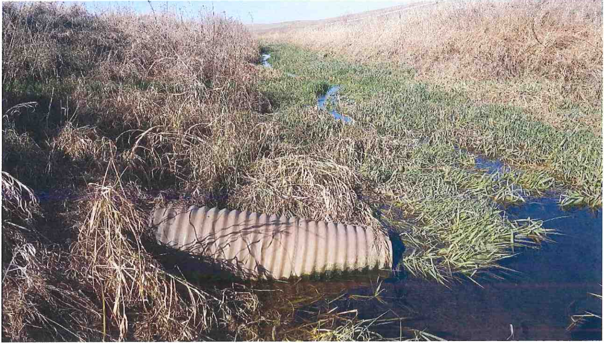
Surface drain collapsed into Open Ditch. Open Ditch heavily silted and meandering.
