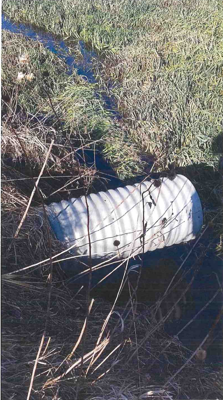
←Surface drain protruding into Open Ditch, lack of support beneath. Open Ditch heavily silted.
