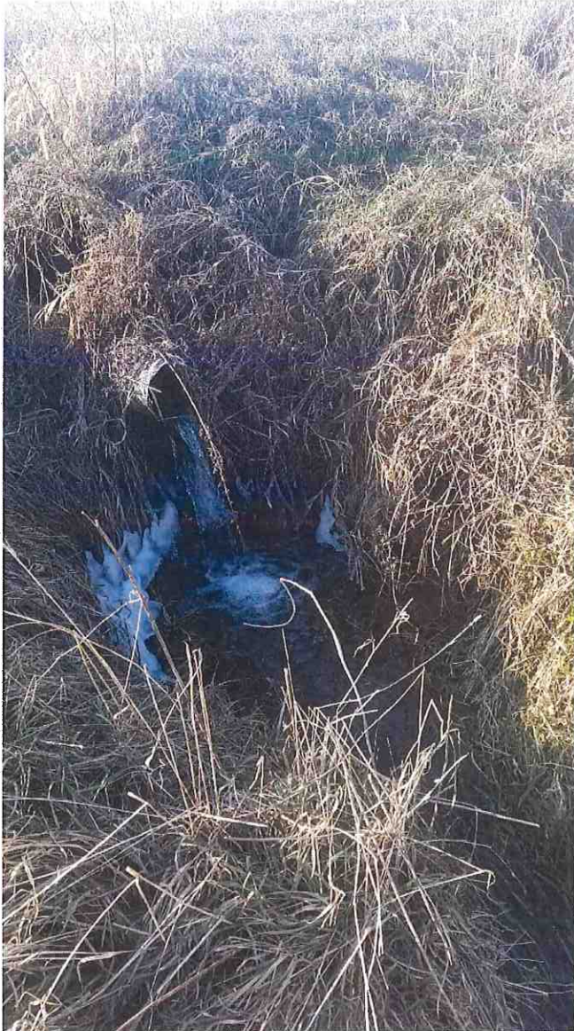
←Tile outlet near Sta. 18+25 +/- cut 8' into bank and causing erosion.
