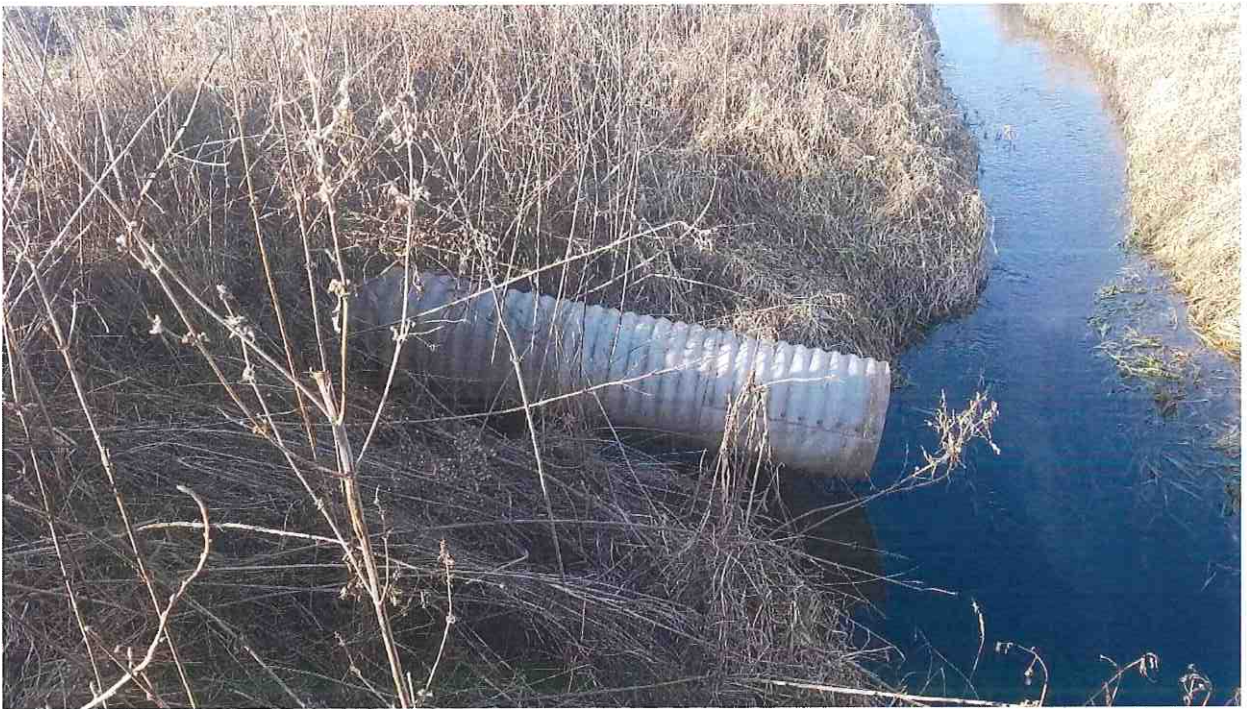
Surface drain with no support beneath near Sta. 23+00 +/-.
